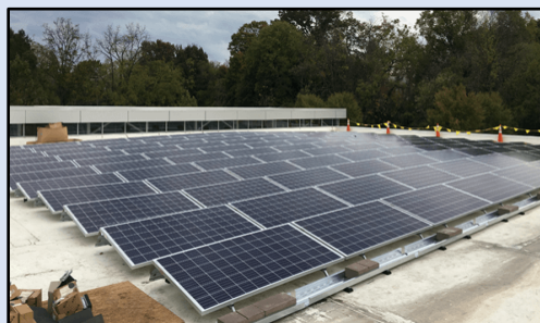
Image 15: Solar PV system on the roof of Smith Aquatics Center.
